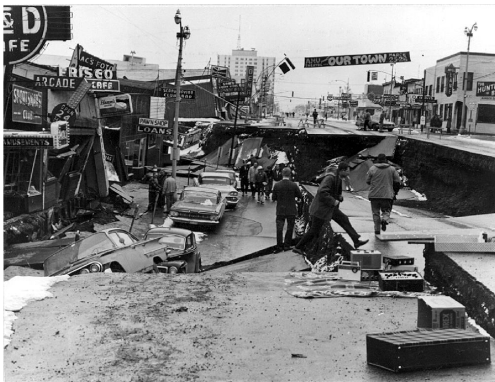
Damage to Fourth Avenue in Anchorage, Alaska caused by the 1964 "Good Friday earthquake." Before the shock, the sidewalk on the left, which is in the graben, was at street level on the right. The graben subsided 11 feet in response to 14 feet of horizontal movement.
